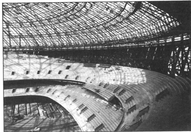
The upper levels of seats rest on concrete decking at the Superdome while ground level stands roll in and out for different sports.
